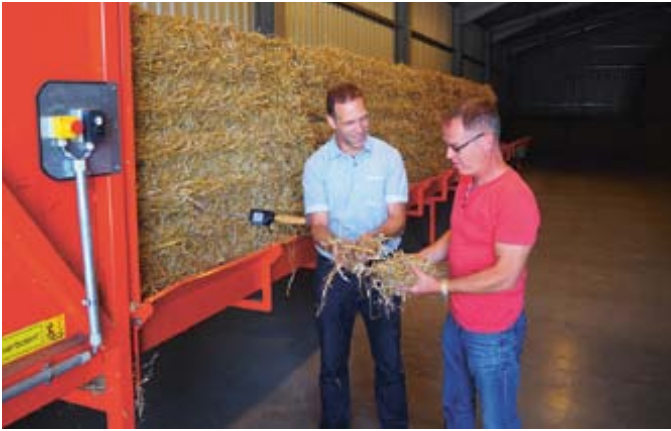
Pilot-Strohheizungsanlage in Gülzow, Mecklenburg-Vorpommern
